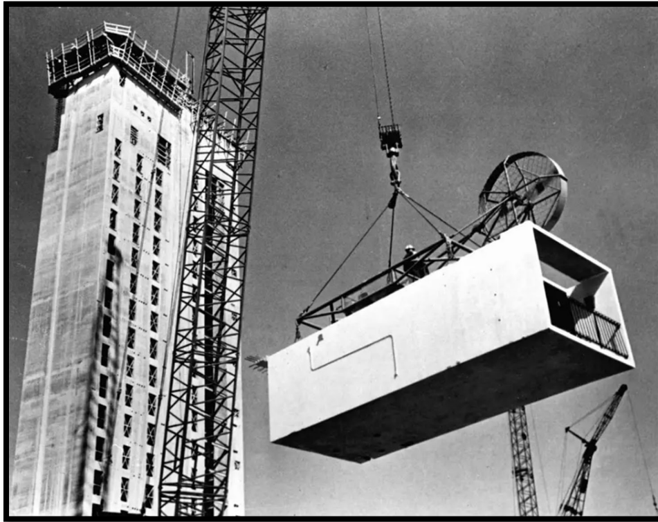
Zachry crews lift a prefabricated room to stack it onto the Hilton Palacio del Rio on the River Walk in 1967.
