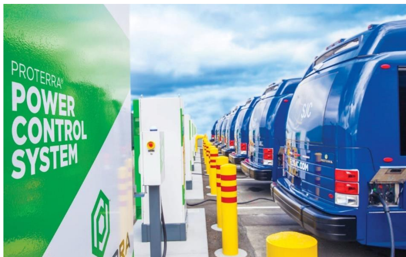
Proterra’s charging infrastructure allows charging up to 20 vehicles simultaneously.
