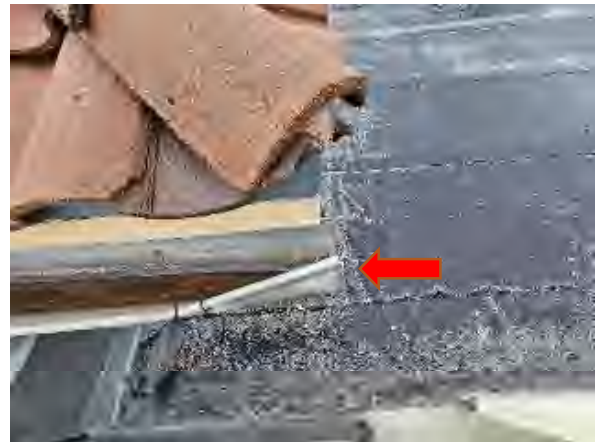
Syedi #32 View of damaged gutter
