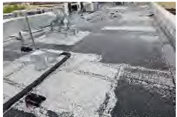
Syedi #6 Original Plaza Bldg.: Many patches/repairs
