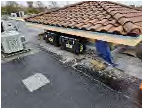
Hull #1 Building materials and debris observed on the roof.
