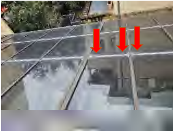
Syedi #49 Greenhouse: Sealant starts deterioration
