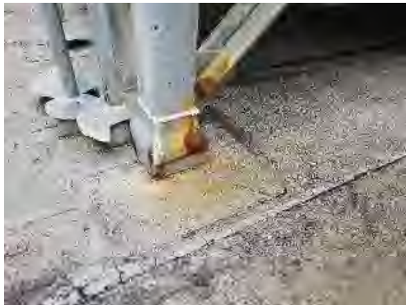
Syedi #47 Cooling Tower: Pitch pan shows rusting/deterioration
