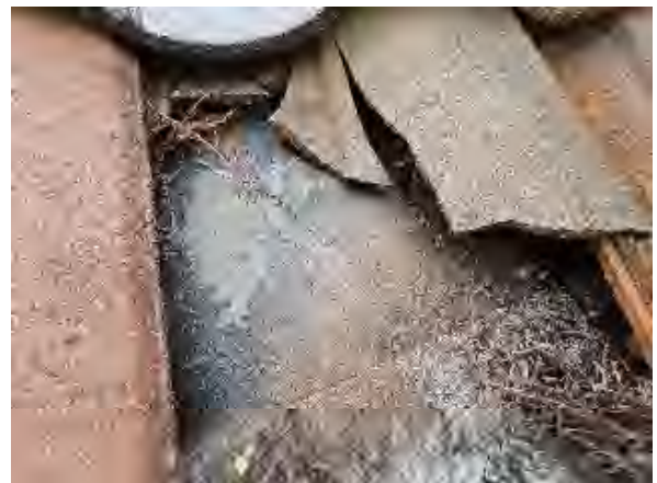
Syedi #30 View of broken tiles on roof. Located periodically through site
