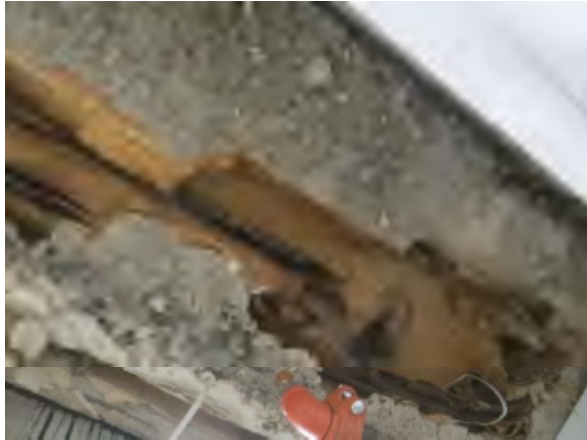
Flores #13 Overview of active water infiltration at EJ observed during our site visit from storage area.
