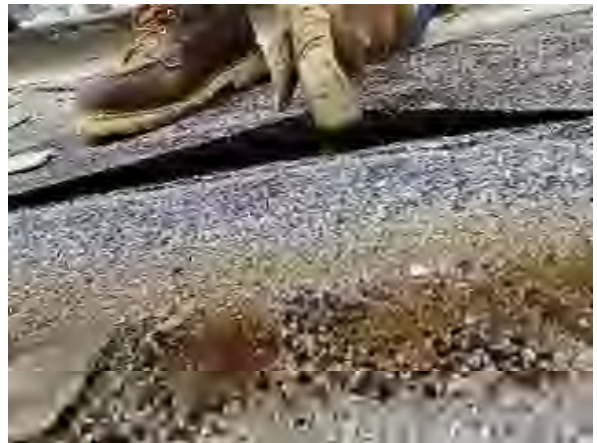
Syedi #46 Cooling Tower: Separation/defects seams
