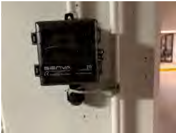
Freeman #3 Basement Parking Area. Wall Mounted Toxic Gas Sensor. Not Operating
