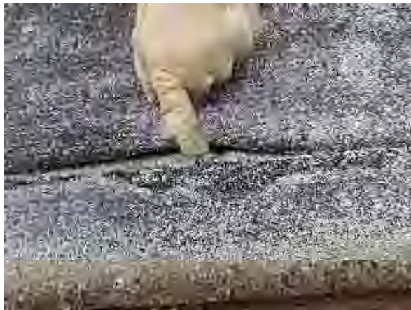
Syedi #45 Cooling Tower: Separation/defects seams
