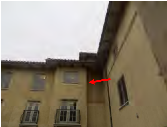
Flores #1 Overview of EJ observed from courtyard (arrow)
