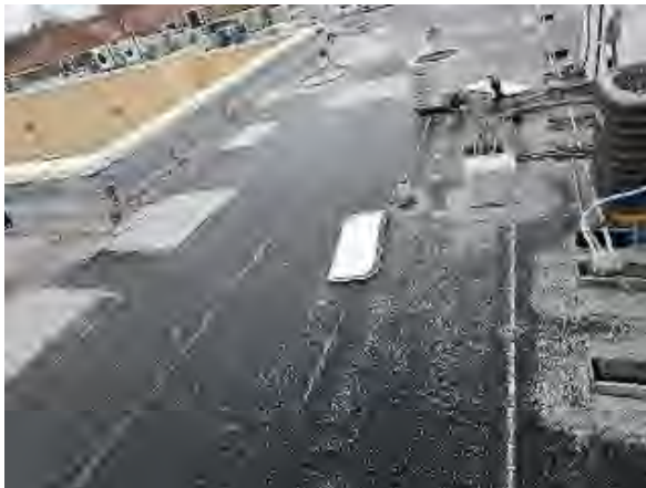
Syedi #3 Original Plaza Bldg.: Many patches/repairs
