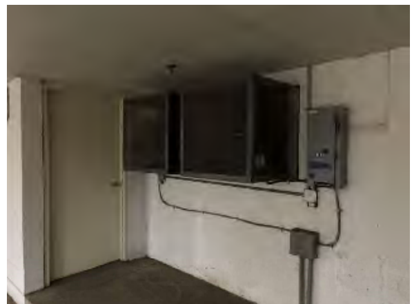
Freeman #18 Phase II Parking Area, Garage Exhaust Fans – Not Operating
