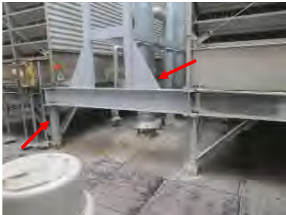
Flores #17 Overview of apparent newly painted hot-rolled steel at the cooling tower. View of the front near the access door. (arrows).
