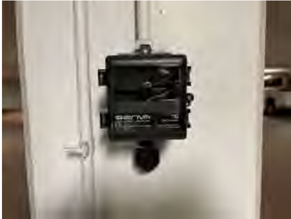
Freeman #1 Basement Parking Area, Wall Mounted Toxic Gas Sensor. Not Operating
