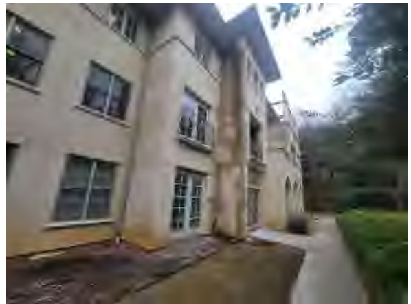
Williams #28 Wet Walls, Building #6 south elevation
