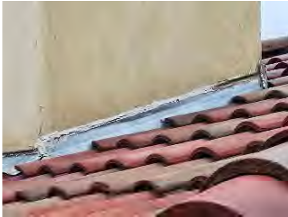
Syedi #43 Improper flashing repair at the base of chimney
