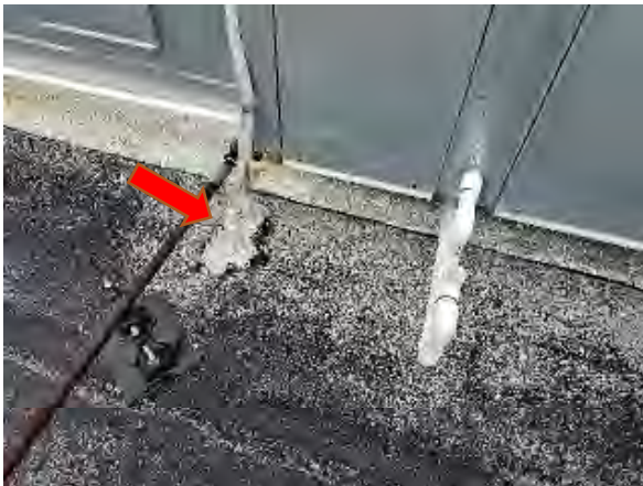
Syedi #41 Not a proper pipe flashing detail
