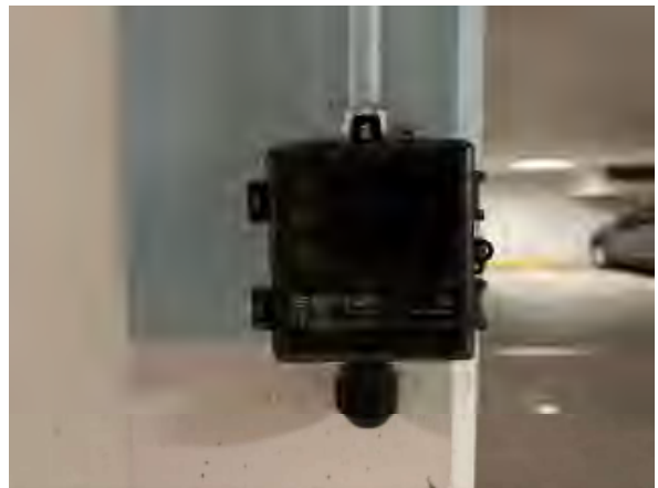
Freeman #10 Phase I Parking Area, Wall Mounted Toxic Gas Sensor. Not Operating (Continuation of #9)
