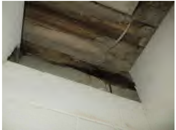
Flores #16 Overview of active water infiltration at EJ observed during our site visit from storage area.
