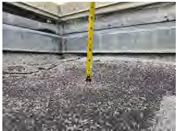
Syedi #18 Original Plaza Bldg.: View of blisters (raised surface areas over voids in the roof system)
