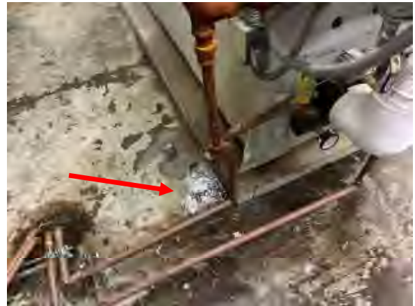
Freeman #32 Central Plant, Existing auxiliary hot water boiler leaking from equipment case.
