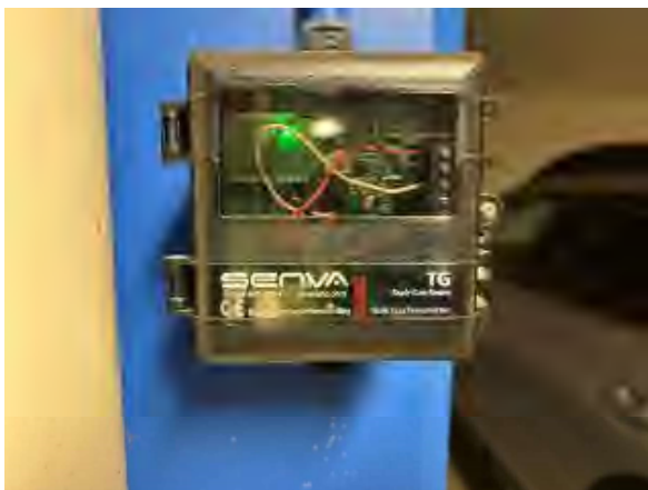
Freeman #17 Phase II Parking Area, Wall Mounted Toxic Gas Sensor. – Not Dual Gas
