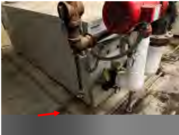
Freeman #33 Central Plant, Existing auxiliary hot water boiler leaking from copper piping.
