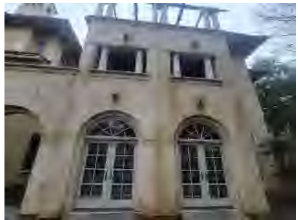
Williams #24 Wet walls, Building #8 south elevation
