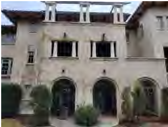
Williams #27 Wet Walls, Building #6 south elevation
