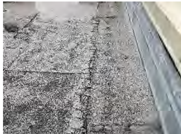
Syedi #22 Original Plaza Bldg.: View of cracking in modified bitumen membrane
