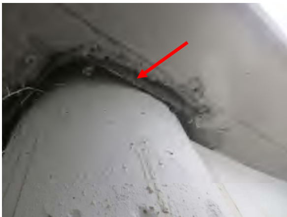
Flores #11 Storage area showing slab poured around existing pier. Note exposed rebar (arrow.)
