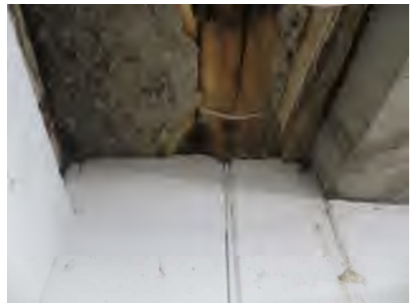
Flores #12 Overview of active water infiltration at EJ observed during our site visit from storage area.
