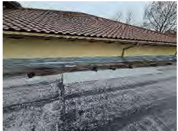
Syedi #8 West Commons Corridor: Many patches/repairs
