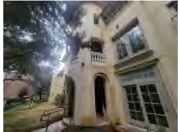
Williams #32 Wet Walls, Building #4 south elevation
