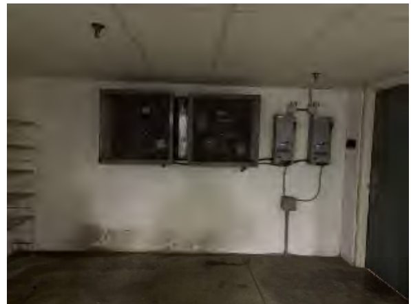
Freeman #16 Phase II Parking Area, Garage Exhaust Fans – Not Operating
