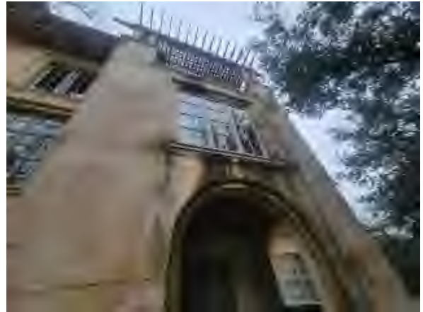
Williams #14 Wet walls, Building #9 west elevation Courtyard
