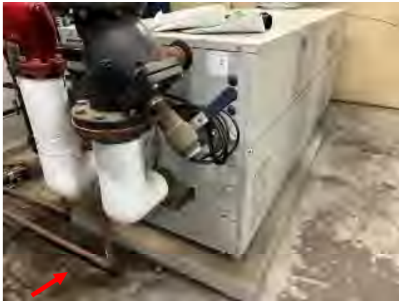
Freeman #31 Central Plant, Existing auxiliary hot water boiler leaking from equipment case.
