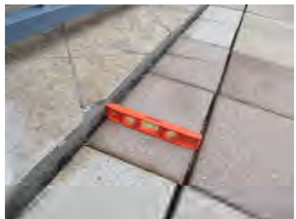
Flores #6 Overview of distress at the pavers from courtyard observed at the courtyard.
