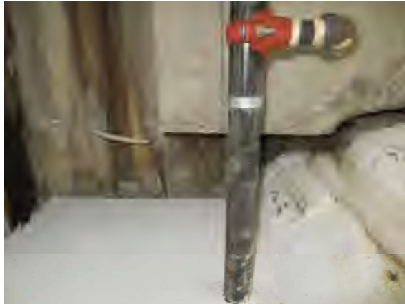
Flores #15 Overview of active water infiltration at EJ observed during our site visit from storage area.
