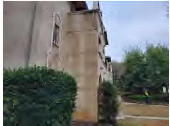
Williams #26 Wet Walls, Building #6 south elevation
