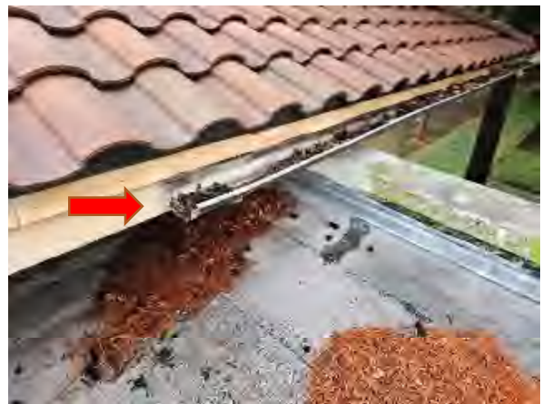
Syedi #34 View of missing gutter piece and gutter clogged with debris
