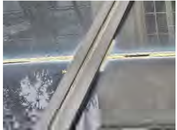
Syedi #50 Greenhouse: Close-up view of deteriorated sealant
