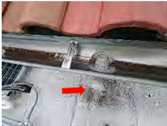
Syedi #31 View of gutter with no downspout and splash block
