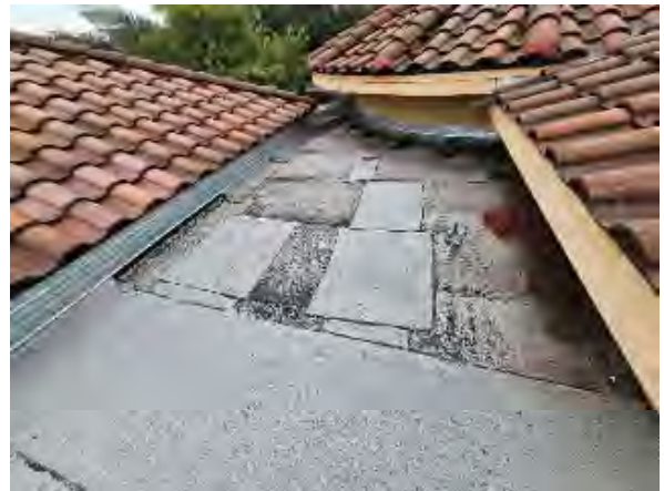
Syedi #10 East Commons Corridor: Many patches/repairs have been noticed
