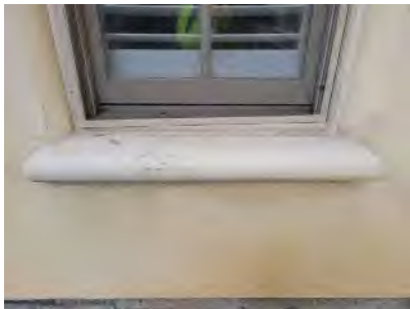
Williams #47 Close-up of hail damaged/deteriorated windowsill on south elevation of Building #8. Several on L1 along this elevation
