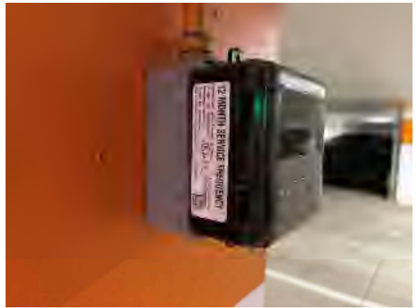
Freeman #20 Phase II Parking Area, Wall Mounted Toxic Gas Sensor, Model No. TGW-ACX-A Not Dual Gas (Continuation of #19)
