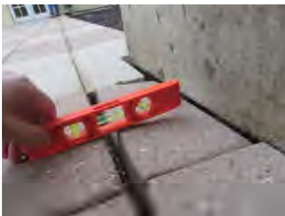
Flores #5 Overview of distress at the pavers from courtyard observed at the courtyard.
