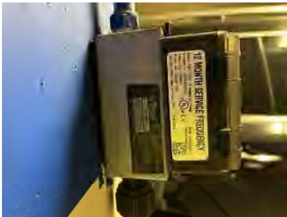
Freeman #15 Phase I Parking Area, Wall Mounted Toxic Gas Sensor, Model No. TGW-ACX-A – Not Dual Gas (Continuation of #14)
