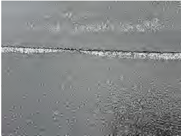
Syedi #13 Original Plaza Bldg.: Separation/defects seams
