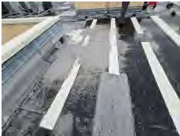
Syedi #11 Original Plaza Bldg.: Patches/repairs along the seams
