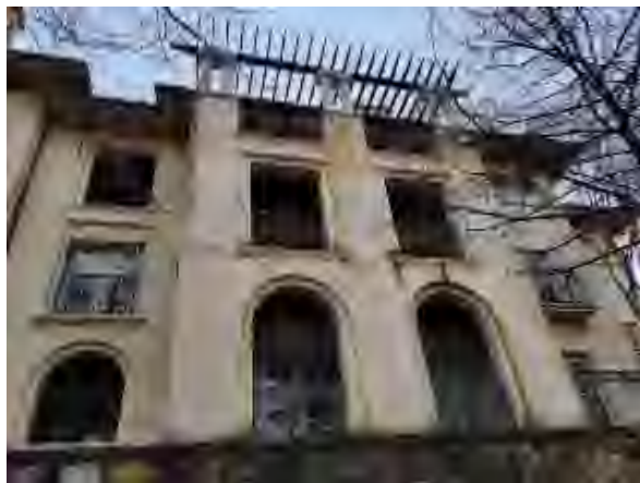
Williams #11 Wet walls, Building #9 Fountains Courtyard
