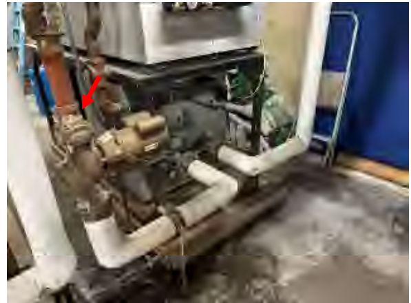
Freeman #26 Copper Piping, severe electrolysis corrosion
