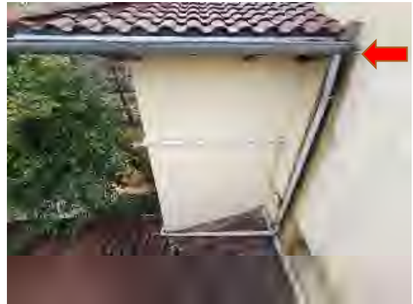
Syedi #38 View of water staining to wall surface from gutter
