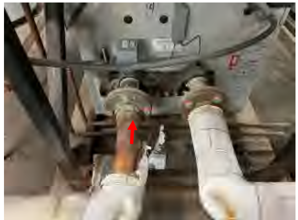
Freeman #24 Copper Piping, severe electrolysis corrosion
