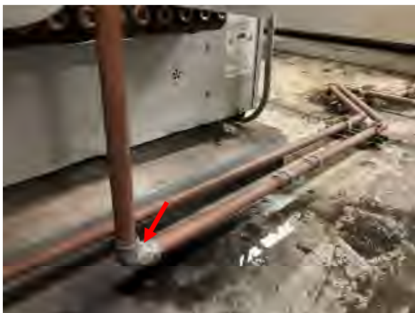
Freeman #29 Copper Piping, Leaking joint. Appeared to be repaired with silver tape.
