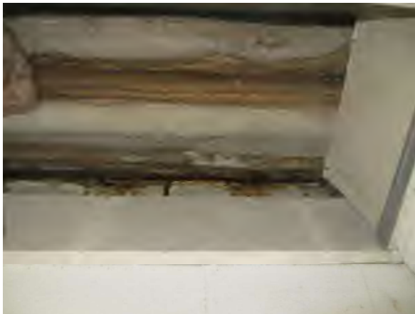
Flores #9 Overview of active water infiltration at EJ observed during our site visit at drive aisle. Tile was missing and water drips were observed.
