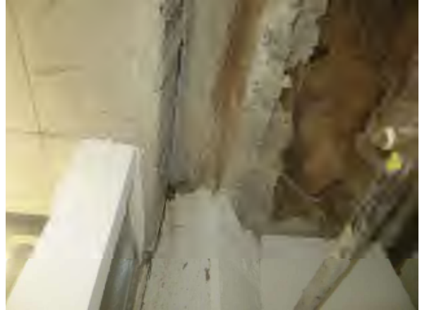
Flores #14 Overview of active water infiltration at EJ observed during our site visit from storage area.
