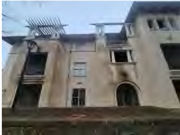
Williams #7 Wet walls, Building #3 PAC Courtyard
