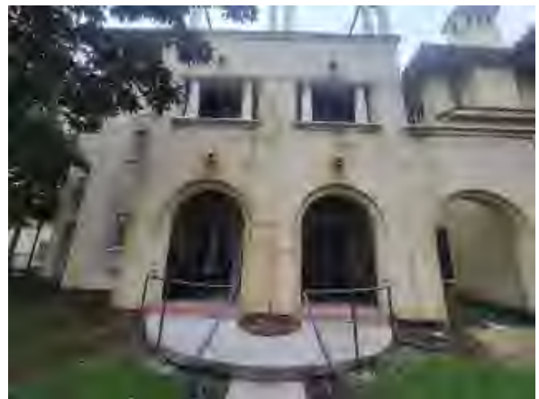
Williams #30 Wet Walls, Building #4 south elevation
