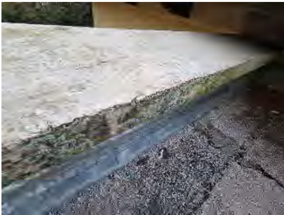
Syedi #51 View of damage to EIFS coping
