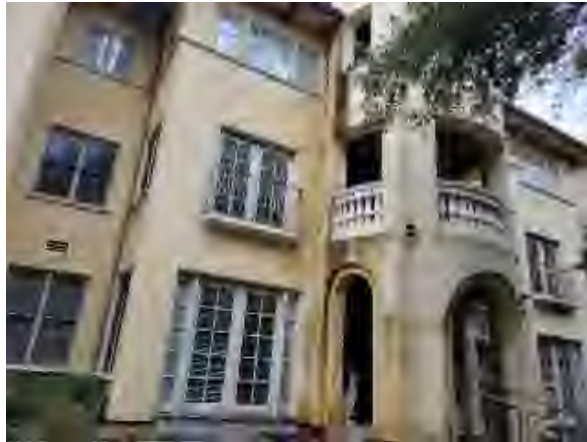
Williams #31 Wet Walls, Building #4 south elevation
