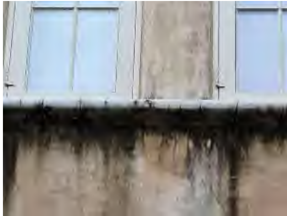
Williams #37 Close-up of badly deteriorated EPS belt course in the east courtyard at Plaza Building. Typical condition this building. .
