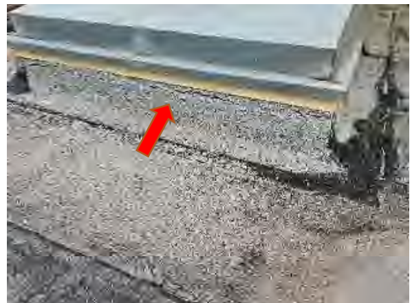
Syedi #24 East Commons Corridor: View of cracking in modified bitumen flashing membrane
