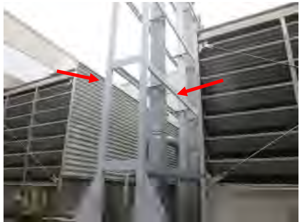
Flores #18 Overview of apparent newly painted hot-rolled steel at the cooling tower. View of the front near the access door. (arrows).
