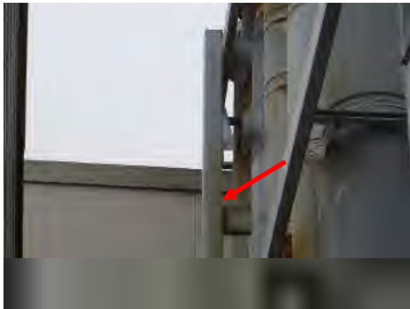
Flores #21 Overview of apparent old hot-rolled steel paint at the cooling tower. View of the rear steel. Arrow indicates heavy oxidation and rust stains.
