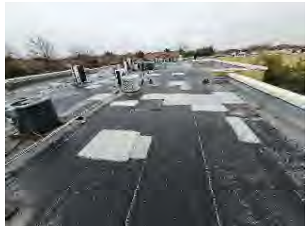
Syedi #4 Original Plaza Bldg.: Many patches/repairs
