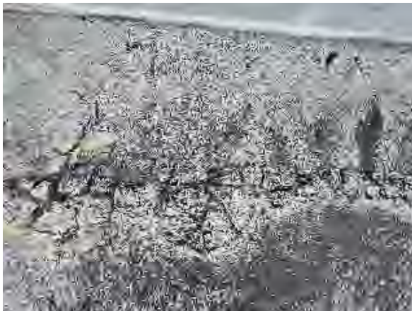
Syedi #21 Original Plaza Bldg.: View of cracking in modified bitumen membrane
