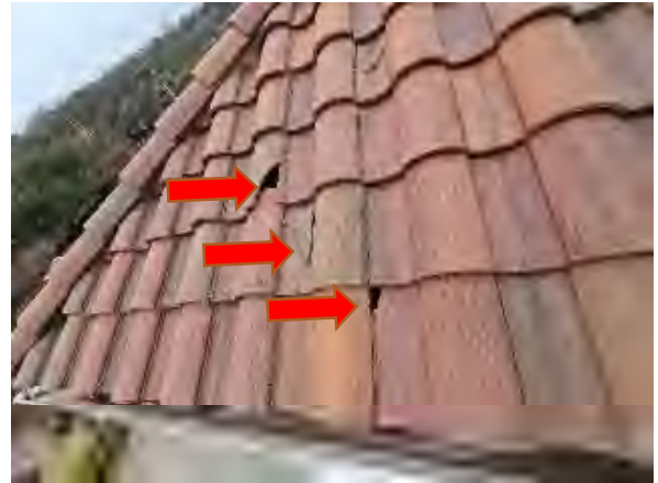
Syedi #26 View of broken tiles on roof. Located periodically through site
