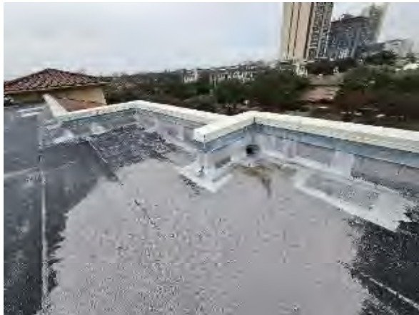
Syedi #7 West Commons Corridor: Many patches/repairs
