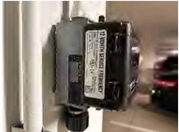
Freeman #2 Basement Parking Area, Wall Mounted Toxic Gas Sensor, Model No. TGW-ACX-A – Not Dual Gas / Not Operating (Continuation of #1)
