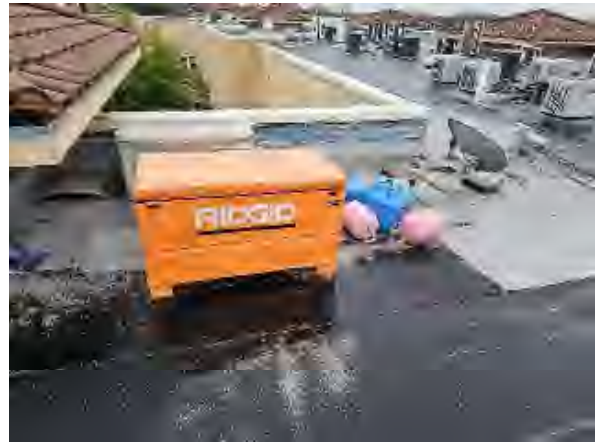
Hull #2 Building materials and debris observed on the roof.
