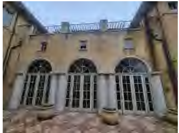
Williams #10 Wet walls, Building #9 Fountains Courtyard
