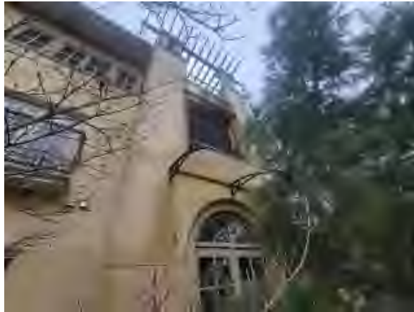
Williams #13 Wet walls, Building #9 north elevation Courtyard
