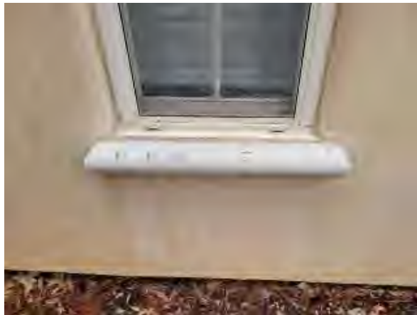
Williams #45 Close-up of hail damaged windowsill on the south elevation at The Plaza in the Putting Green Courtyard
