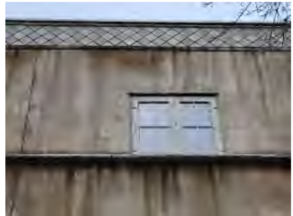
Williams #46 Close-up of badly deteriorated EPS belt course and molding below tile on the east elevation of The Plaza Building. .
