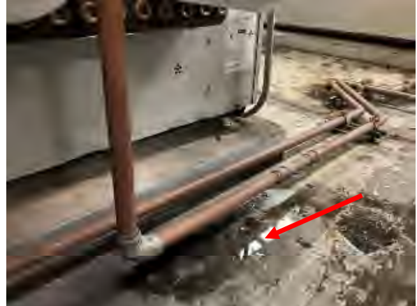
Freeman #34 Central Plant, Existing auxiliary hot water boiler leaking from copper piping.
