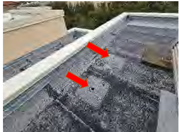
Syedi #42 The height of existing vent stack pipes doesn't meet the international plumbing code (IPC) requirements (8" min. flashing height)
