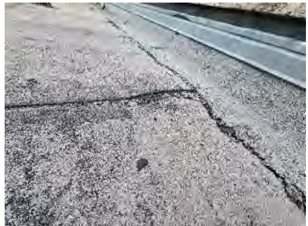
Syedi #20 East Commons Corridor: View of blisters (raised surface areas over voids in the roof system)
