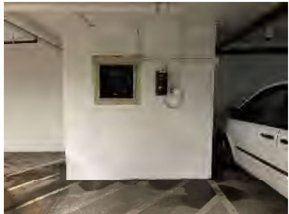
Freeman #4 Plaza Parking Area, Operational Garage Exhaust Fan
