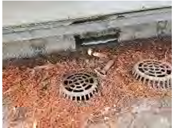
Syedi #44 View of roof drain clogged with debris
