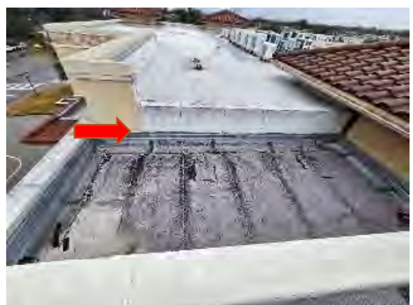
Syedi #54 South addition to original plaza: No expansion joint was noticed.
