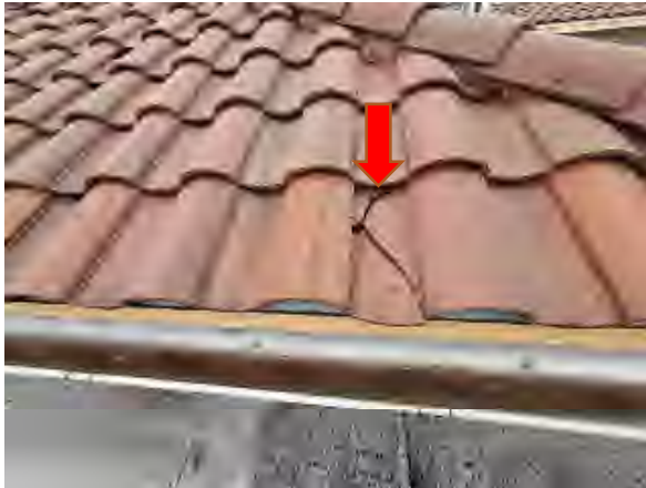
Syedi #25 View of broken tiles on roof. Located periodically through site
