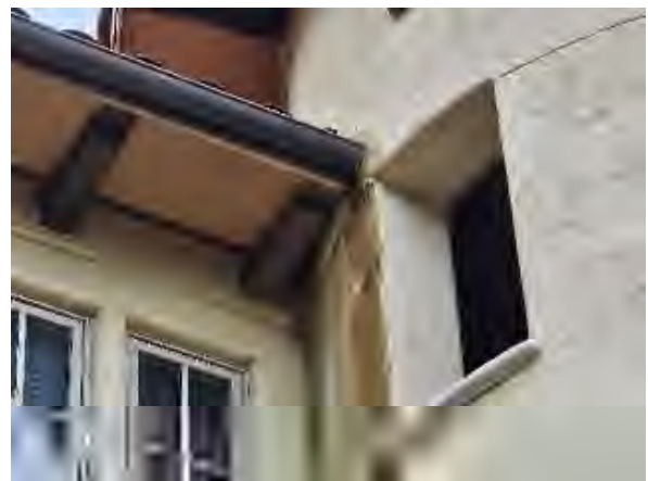
Syedi #36 View of water staining to wall surface from gutter
