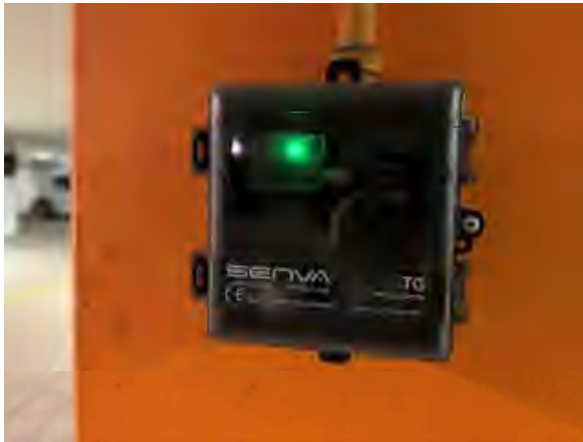
Freeman #19 Phase II Parking Area, Wall Mounted Toxic Gas Sensor
