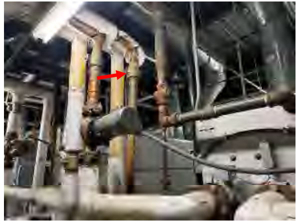
Freeman #22 Copper Piping, severe electrolysis corrosion
