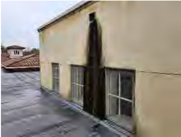
Syedi #39 View of water staining to wall surface from scupper
