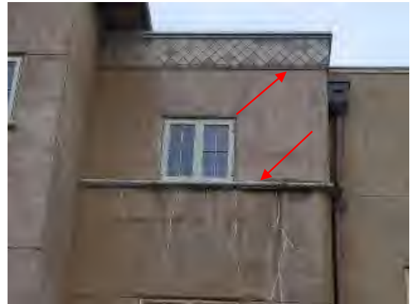
Williams #44 Close-up of deteriorated EPS belt course and molding below tile on the west elevation of The Plaza Building. .
