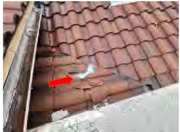
Syedi #28 View of broken tiles on roof. Located periodically through site
