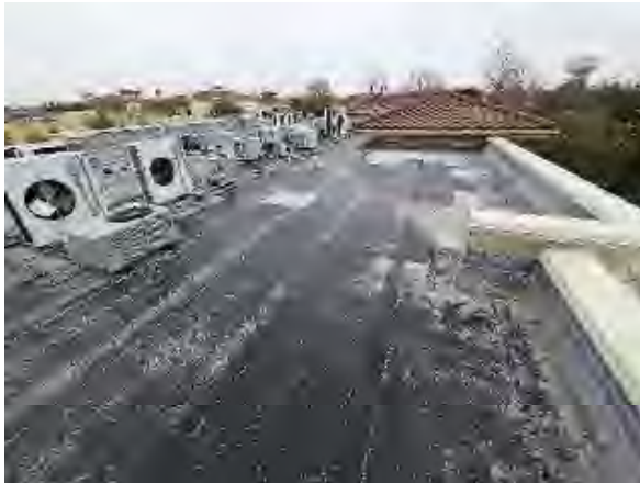
Syedi #1 Original Plaza Bldg.: Roof is in very poor condition, with signs of granule loss at most of the roof membranes
