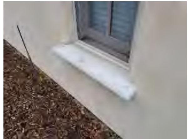
Williams #34 Hail damaged and cracked finish coat EPS windowsill on east elevation at Building #1
