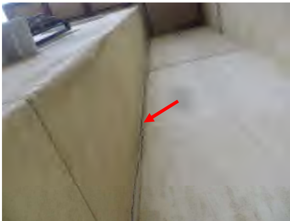
Flores #3 Overview of EJ observed from courtyard. Note separation at joint (arrow)
