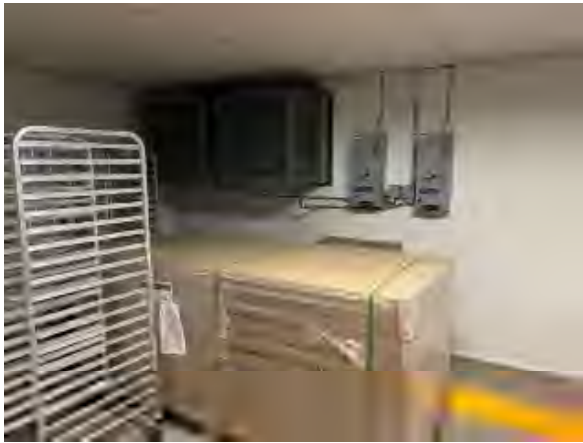
Freeman #21 Phase II Parking Area, Garage Exhaust Fans – Not Operating
