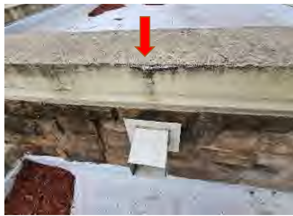
Syedi #52 View of damage to EIFS coping
