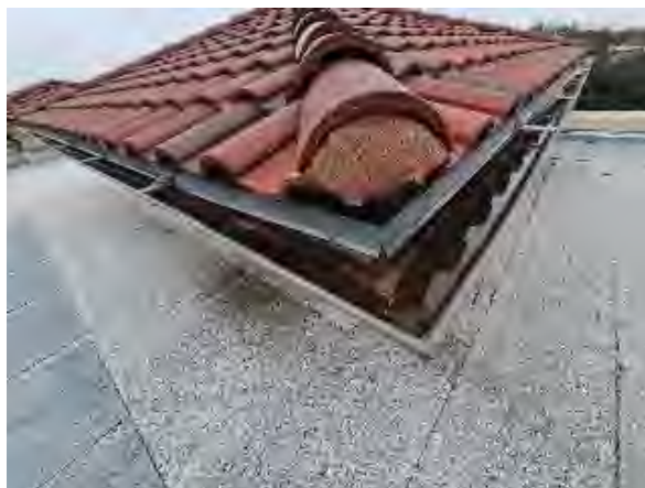
Syedi #35 View of gutter with standing water
