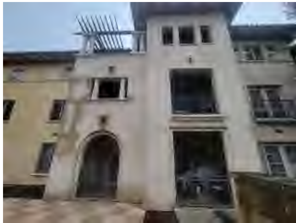
Williams #9 Wet walls, Building #3 Fountains Courtyard
