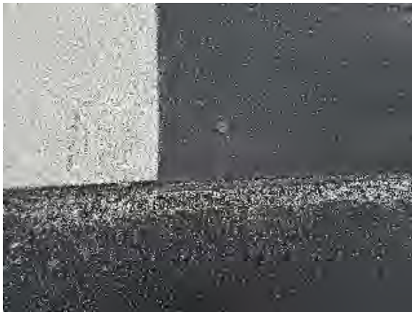
Syedi #15 Original Plaza Bldg.: Shrinkage/separation at the side lap seams
