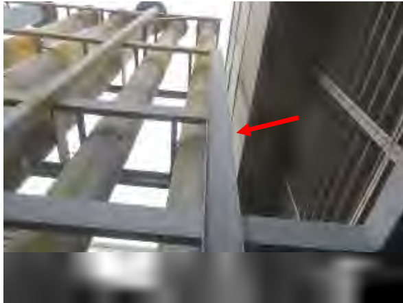
Flores #19 Overview of apparent newly painted hot-rolled steel at the cooling tower. View of the rear steel. Arrow indicates where the fresh paint stops.
