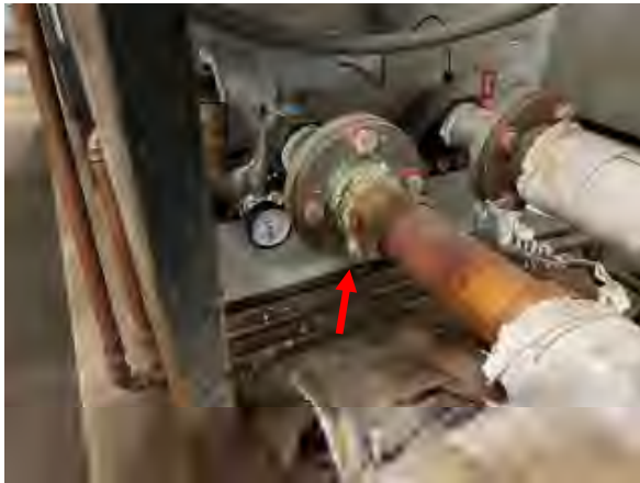
Freeman #25 Copper Piping, severe electrolysis corrosion
