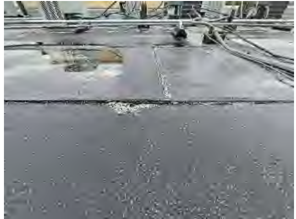
Syedi #14 Original Plaza Bldg.: Separation/defects seams
