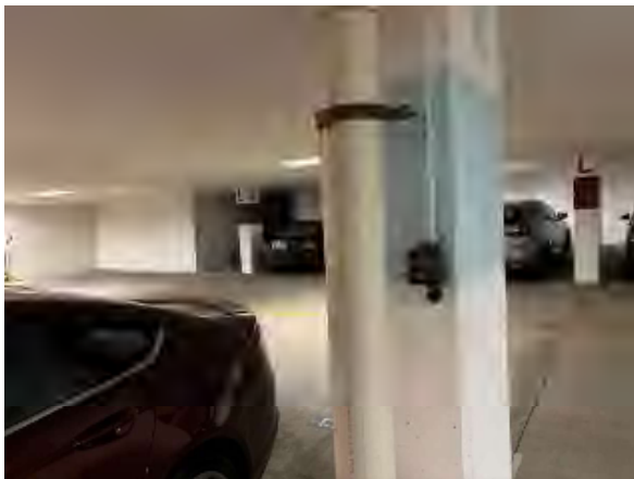
Freeman #9 Phase I Parking Area, Wall Mounted Toxic Gas Sensor
