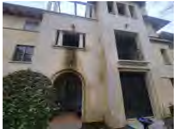
Williams #22 Wet walls, Building 7, west elevation Putting Green Courtyard
