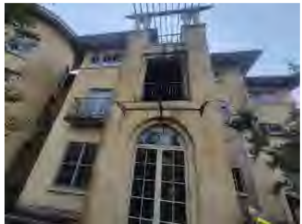
Williams #12 Wet walls, Building #9 north elevation Courtyard
