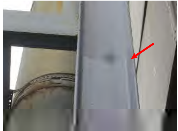
Flores #20 Close-up view of apparent newly painted hot-rolled steel at the cooling tower. View of the rear steel. Arrow indicates where the fresh paint stops. Note oxidation and rust stains to the paint above the arrow.
