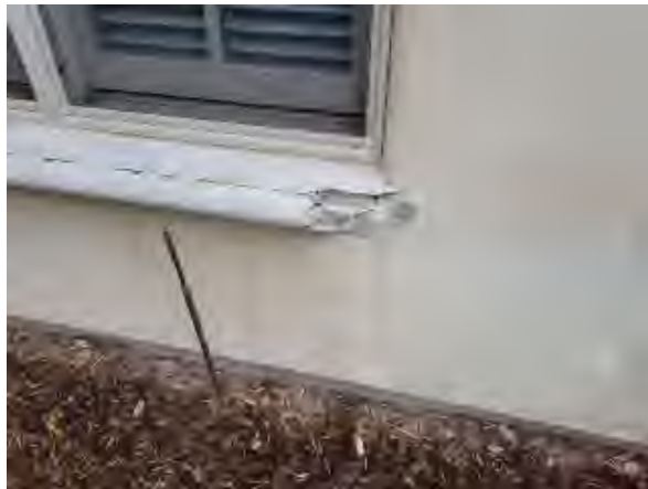
Williams #33 Damaged and deteriorated EPS windowsill with cracked finish coat on east elevation at Building #1
