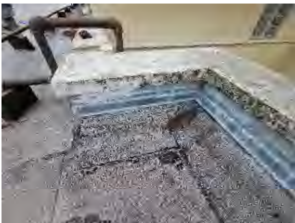
Syedi #23 West Commons Corridor: View of cracking in modified bitumen flashing membrane
