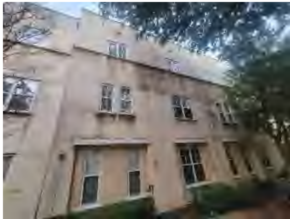
Williams #39 Overview of badly deteriorated EPS windowsill condition in the west courtyard at the Plaza Building. Typical condition this building. .
