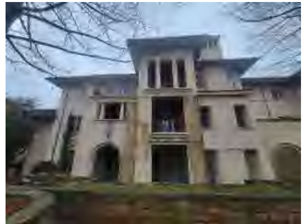
Williams #6 Wet walls, Building #1 PAC Courtyard
