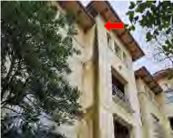
Syedi #37 View of water staining to wall surface from gutter
