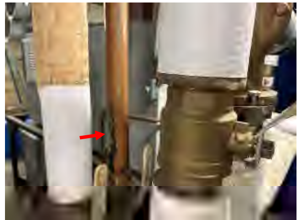
Freeman #28 Copper Piping, severe electrolysis corrosion
