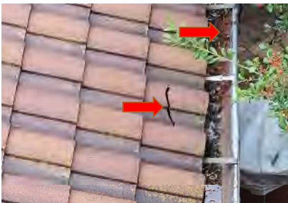
Syedi #29 View of broken tiles on roof and typical gutter clogged with debris. Located periodically through site
