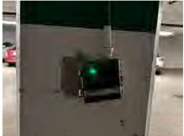
Freeman #8 Plaza Parking Area, Wall Mounted CO/ NO2 Sensor, Model No. TGW-ACN
