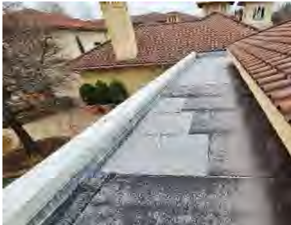
Syedi #9 East Commons Corridor: Many patches/repairs have been noticed
