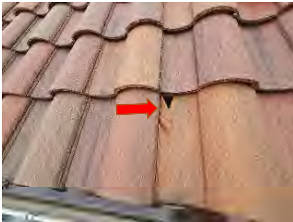
Syedi #27 View of broken tiles on roof. Located periodically through site
