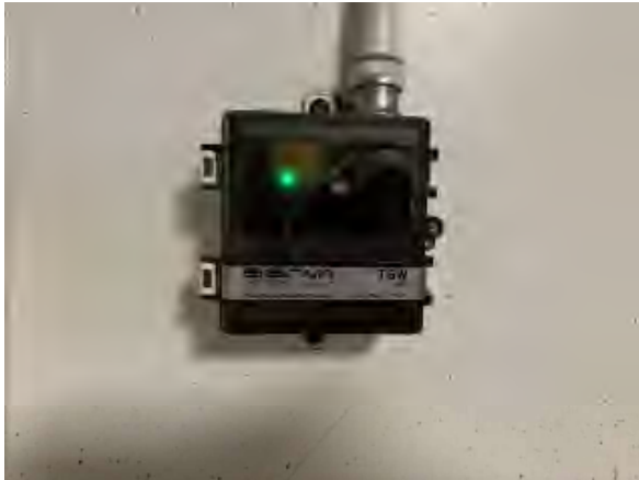
Freeman #7 Plaza Parking Area, Wall Mounted CO/ NO2 Sensor, Model No. TGW-ACN
