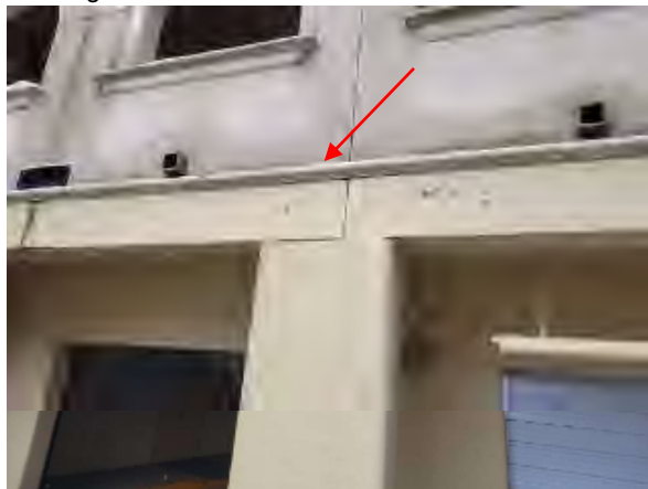
Williams #35 Deteriorated EPS molding with cracked finish coat on north elevation at Building #3
