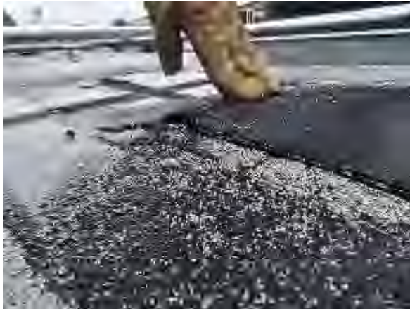
Syedi #19 Original Plaza Bldg.: View of blisters (raised surface areas over voids in the roof system)
