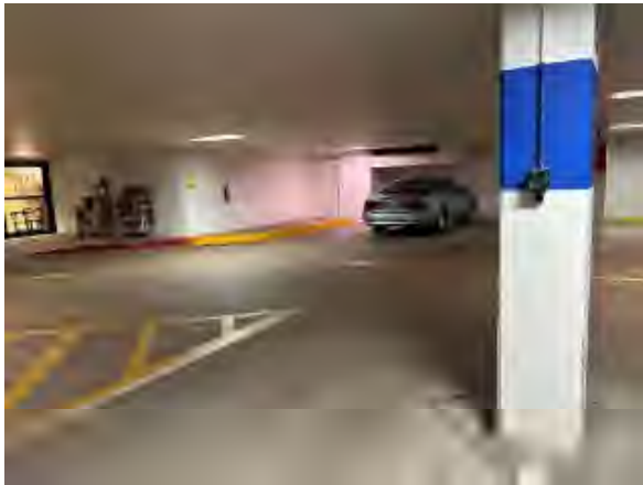
Freeman #13 Phase I Parking Area, Wall Mounted Toxic Gas Sensor
