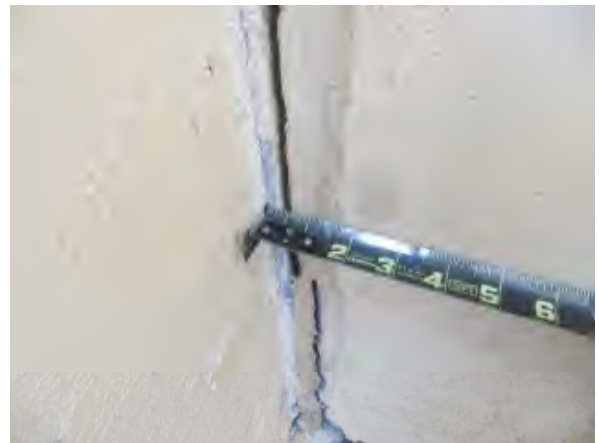
Flores #4 Close-up view of EJ observed from courtyard. Note separation at joint.
