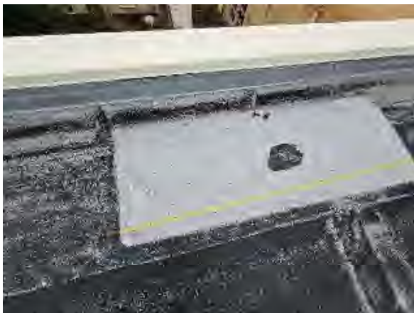
Syedi #5 Original Plaza Bldg.: Many patches/repairs
