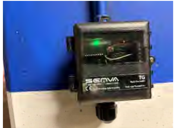
Freeman #14 Phase I Parking Area, Wall Mounted Toxic Gas Sensor
