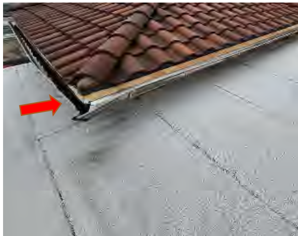
Syedi #33 View of severely damaged gutter
