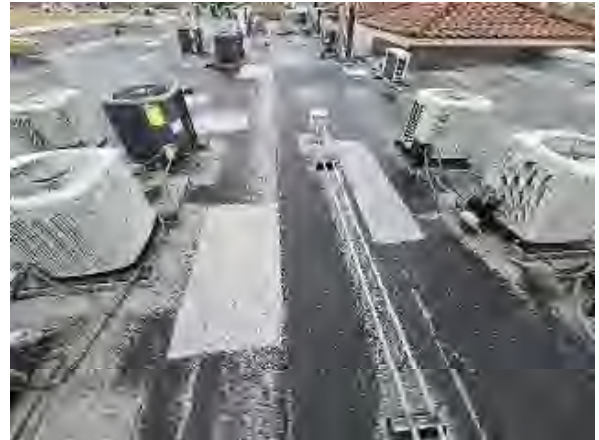
Syedi #2 Original Plaza Bldg.: Many patches/repairs have been noticed
