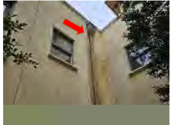
Syedi #40 View of water staining to wall surface from conductor head
