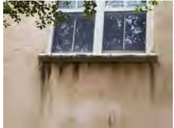
Williams #38 Badly deteriorated EPS windowsill condition in the east courtyard at the Plaza Building. Typical condition this building. .
