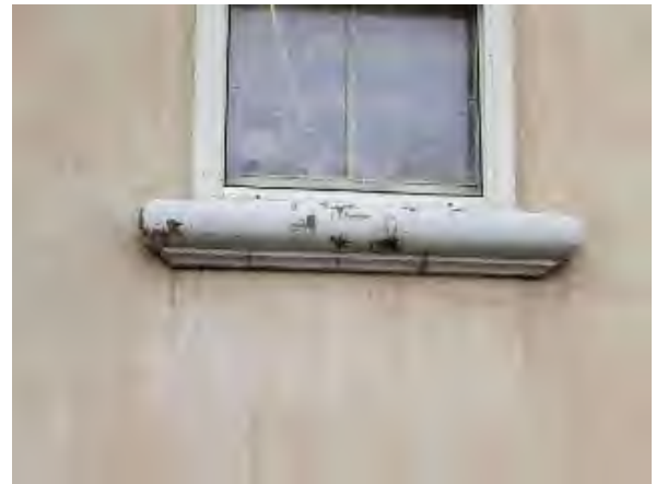
Williams #40 Close-up of hail damaged and deteriorated windowsill on west elevation of the Plaza Building.
