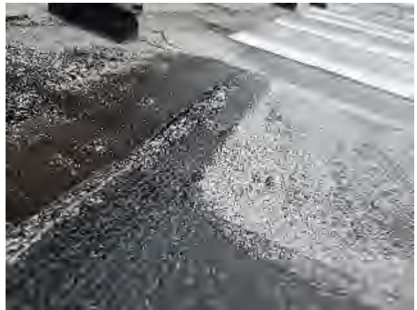
Syedi #16 Original Plaza Bldg.: View of blisters (raised surface areas over voids in the roof system) and separation/defects at the end lap seams
