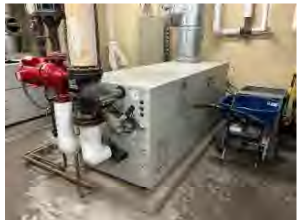
Freeman #30 Central Plant, Existing auxiliary hot water boiler
