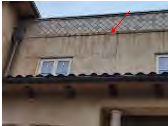
Williams #43 Overview of deteriorated EPS molding below tile on the west elevation of The Plaza Building. .
