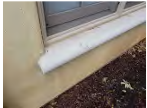
Williams #48 Close-up of damaged windowsill on west elevation of building #5 at Duck Pond Courtyard
