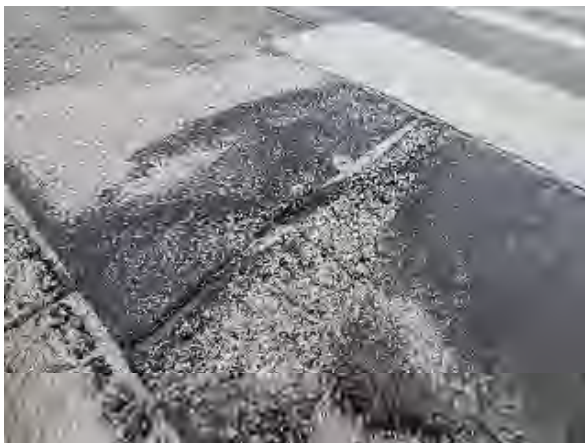
Syedi #17 Original Plaza Bldg.: View of blisters (raised surface areas over voids in the roof system) and separation/defects at the end lap seams
