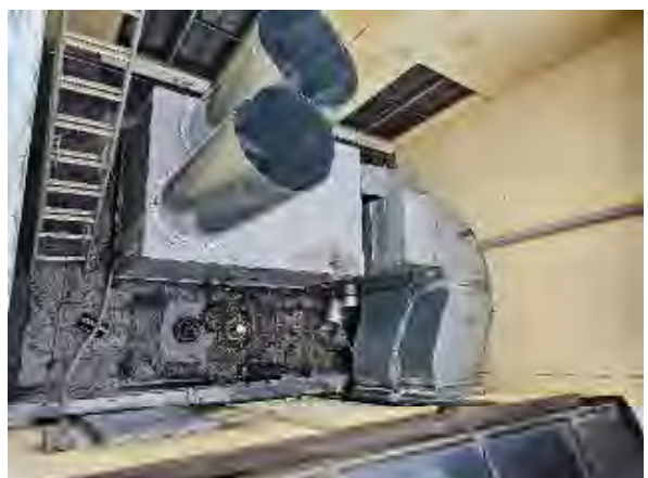
Syedi #48 Greenhouse-RTU room: Roof in poor condition
